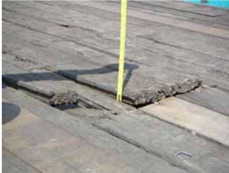
Figure 7 – Damaged plank presenting a trip hazard.
