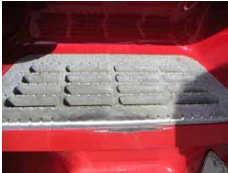
Figure 3 – High levels of wear is usually seen on the outer edges of cab steps.
